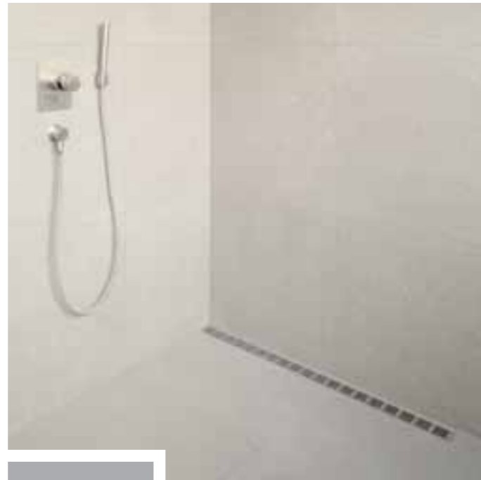
Shower stall with two walls and open/glass wall on right (ClassicLine with Stripe grating)
