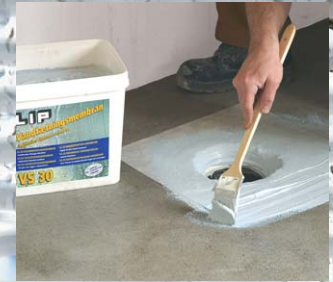
Depending on the type of drainage make sure that all sides are reinforced.
