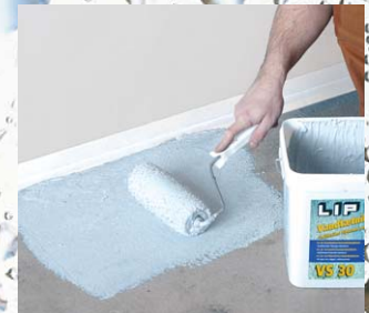
Tanking with LIP VS 30 is easy. 2 layers must be applied to achieve a thickness of 1 mm.
