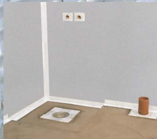
After sealing all joints, corners, pipes ect. the room is ready for priming.
