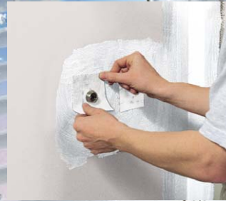
It is very important that the area around the pipes is 100% waterproof as water might run backwards along the pipe into the wall.
